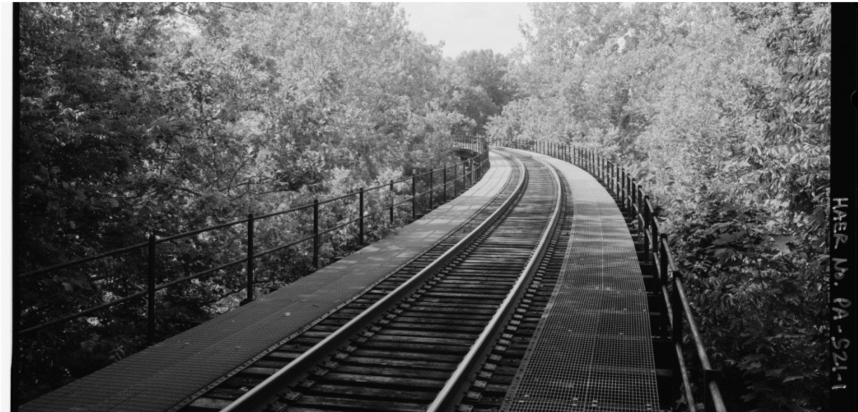
Dramatic View of Pickering Creek Trestle 50' Above State Route 29 and Pickering Creek (Photo from the Historic American Engineering Record)
