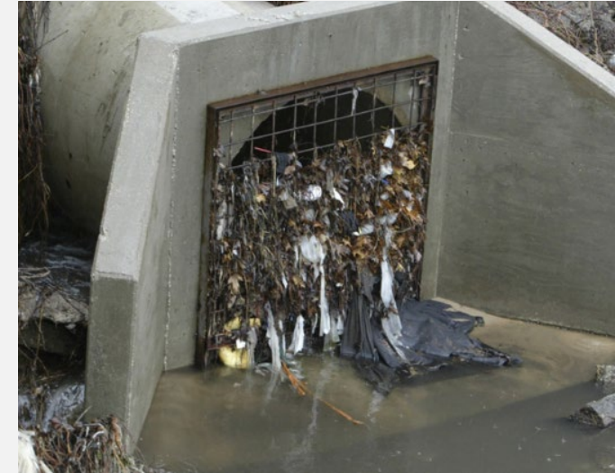
Clogged stormwater drain
